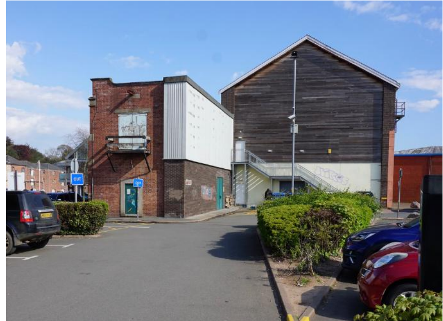
Partial demolition at the north end of the former Electricity Generating Station has resulted in blank frontages and an awkward termination.
