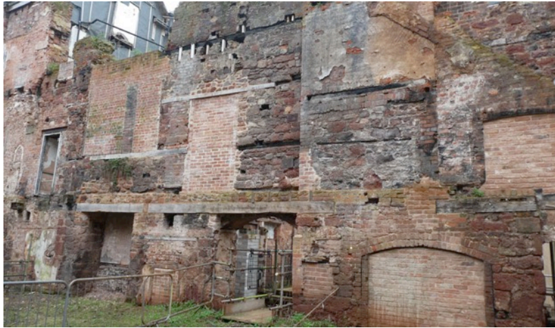
Figure 3. Timber lintels and struts built into saturated exposed masonry walls
