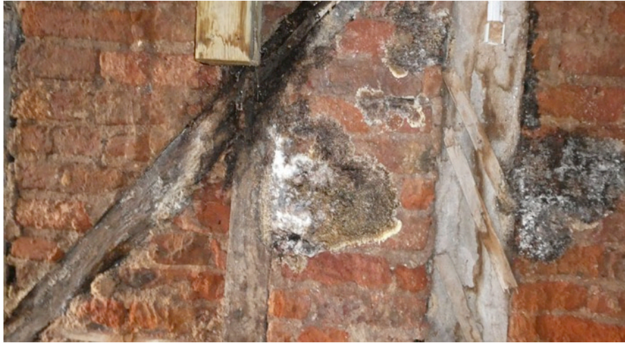
Figure 2. Fungal outbreak on west wall of No.16
