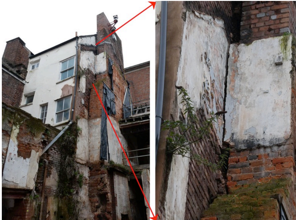
Figure 8. Potentially unstable chimney stack at the north end of site
