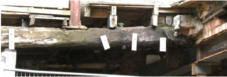
Figure 5. Severe degradation at Location E
