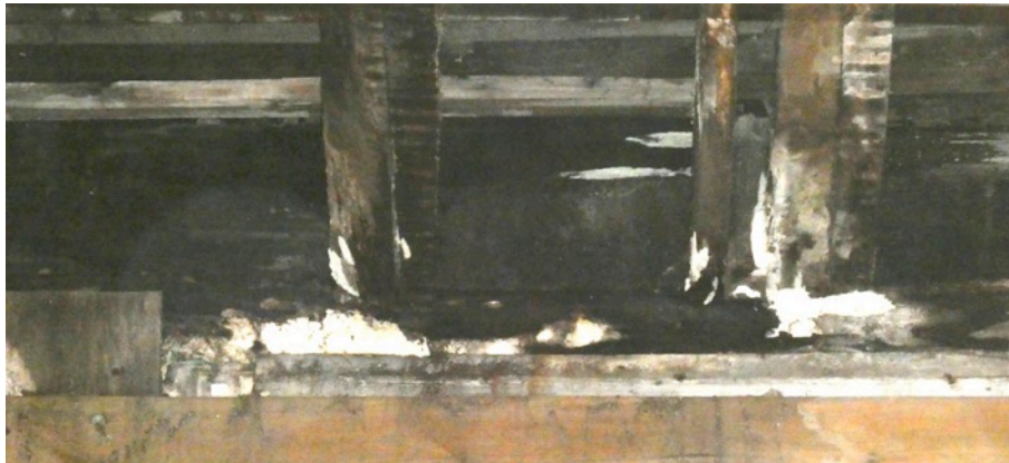
Figure 4. Fungal degradation in first floor timbers
