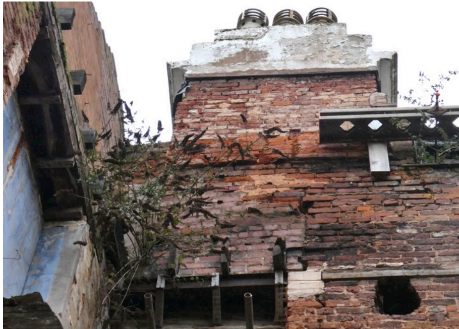
Figure 7. Well established Buddleia bushes growing in the masonry.
