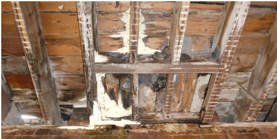
Figure 6. Widespread fungal degradation at Location F
