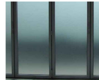
09 - Obscured Window Glazing
