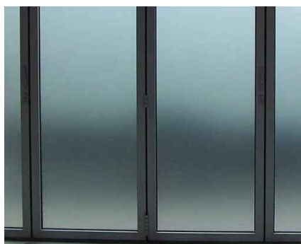
18 - Obscured Window Glazing
