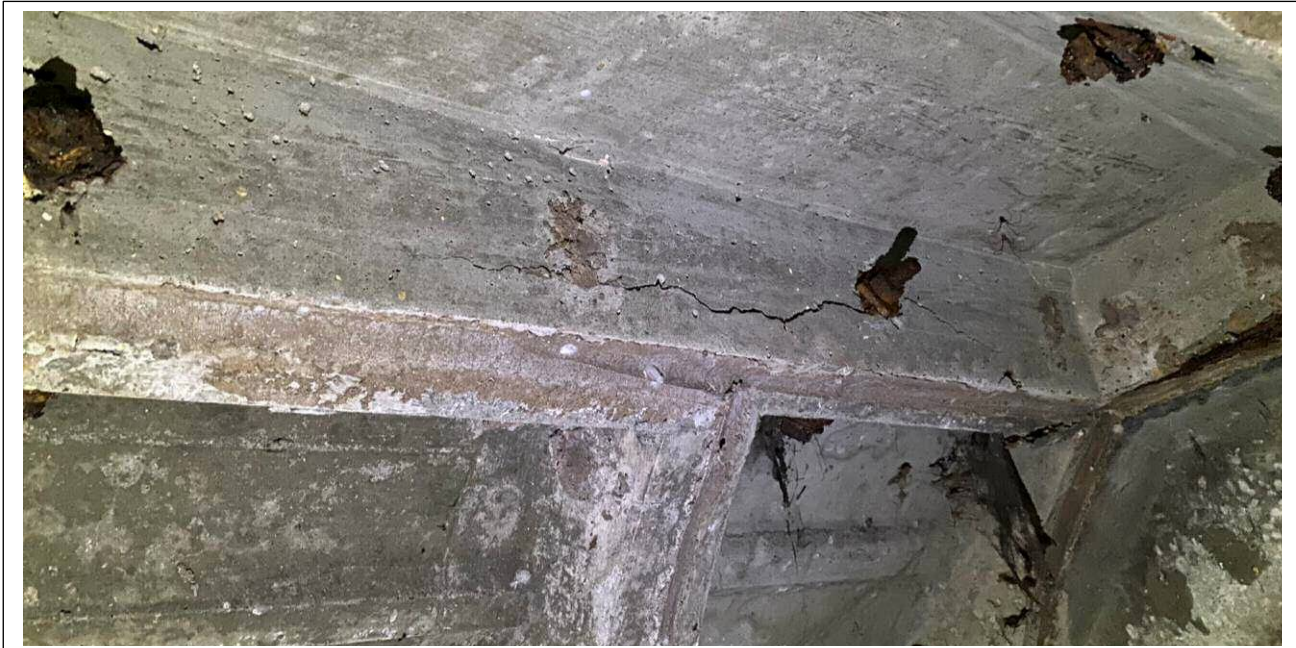
Photo 7 - Surface cracking due to expansion of internal corrosion and bolt corrosion expansion.
