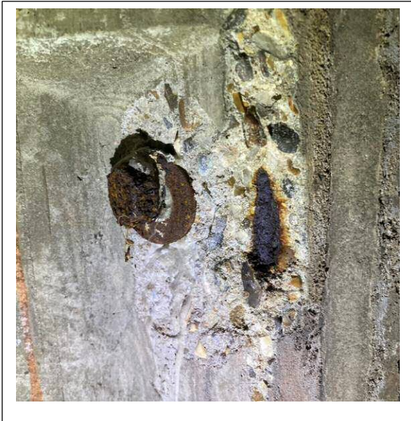
Photo 3 - Corrosion to bolts and effect on surrounding concrete.
