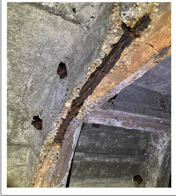
Photo 1 - Primary roof reinforcement exposure and corrosion.
